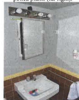
Bathroom interior showing damage to medicine cabinet where Sgt. Jones's round entered and damage to wall where an additional round entered.
