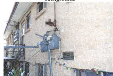
Damage to the brick from a possible round.
